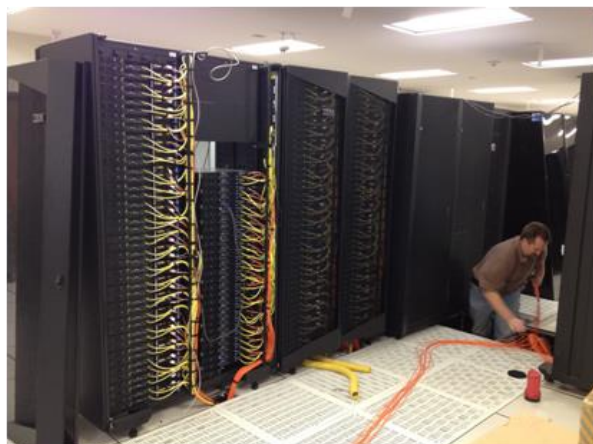
Razor 2 supercomputer installation
